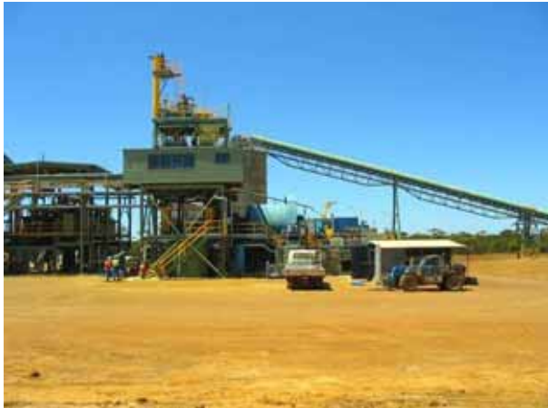
Grinding circuit and control room
