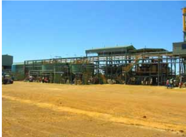
Flotation section on the RHS and concentrate and tailings thickeners on the LHS
